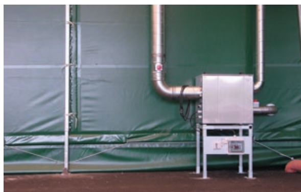
DST dehumidifier Recusorb DR-40 installed in a plastic storage tent.
