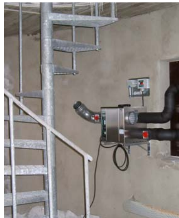
Installed a dehumidifier in the ventilation space in the water tower in Lit. Photograph from Polair.
